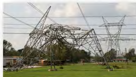
Damaged High Voltage Distribution Tower Credit: FEMA
