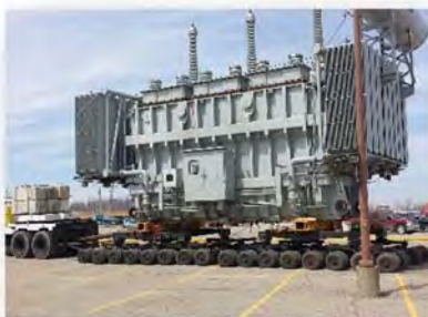
Extra High Voltage Transformer Credit: DTE Energy
